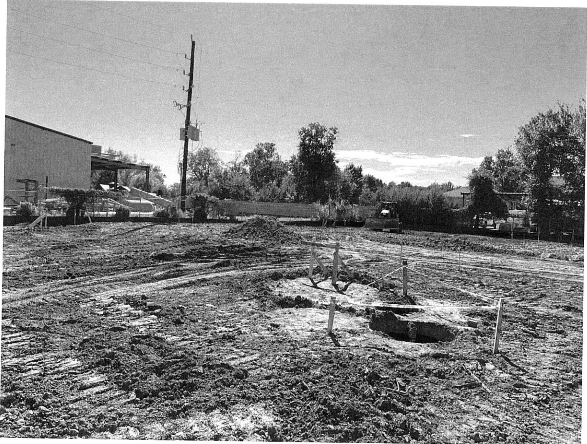
10/9/23 Existing septic tank found outside building pad area (Second tank found next to first subsequently)
